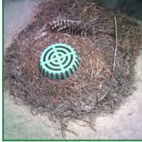
Clogged Drain Systems
